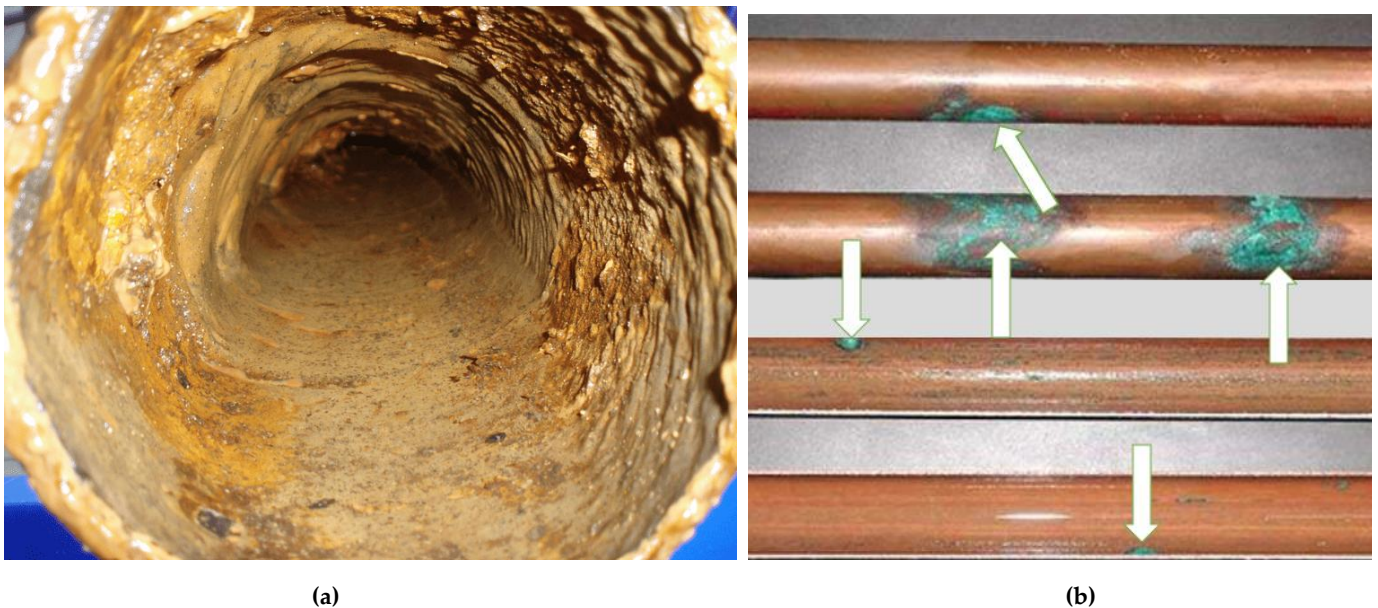
Figure 2. (a) Surface corrosion on a 200 mm (DN 200) steel drinking water pipe after nearly 100 years of operation. (b) Pitting corrosion on copper pipes. Leaks are indicated by white arrows.
